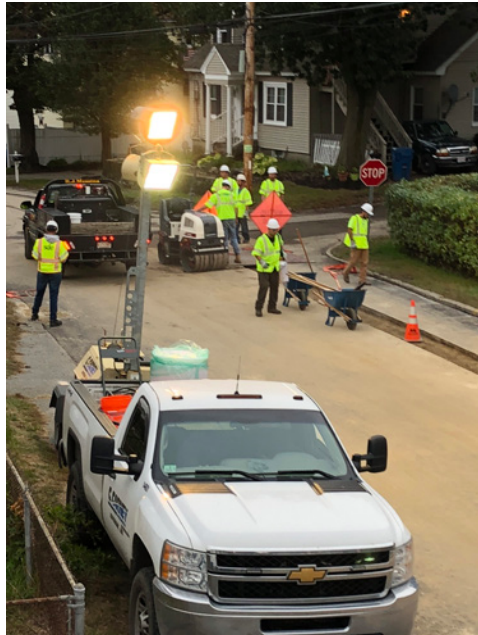
Inspectors working in Lawrence following the gas explosions.
