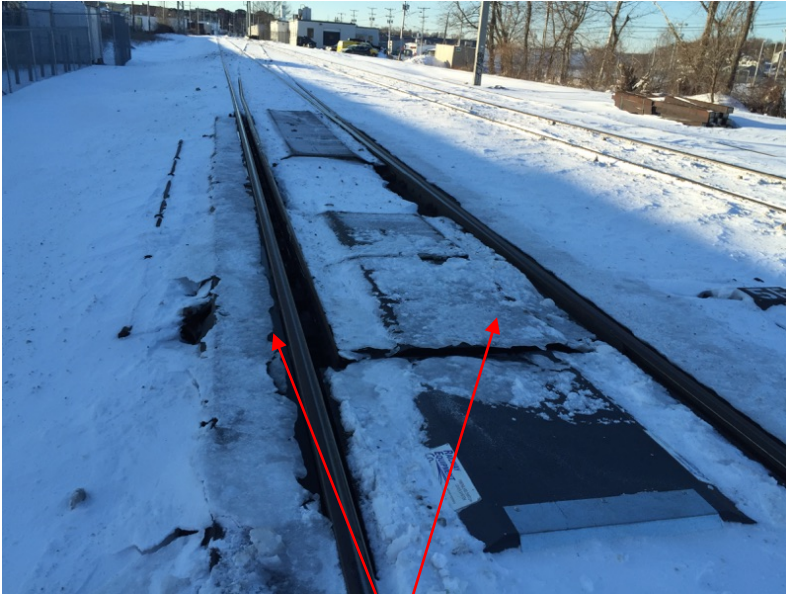
Old Electric Heating
