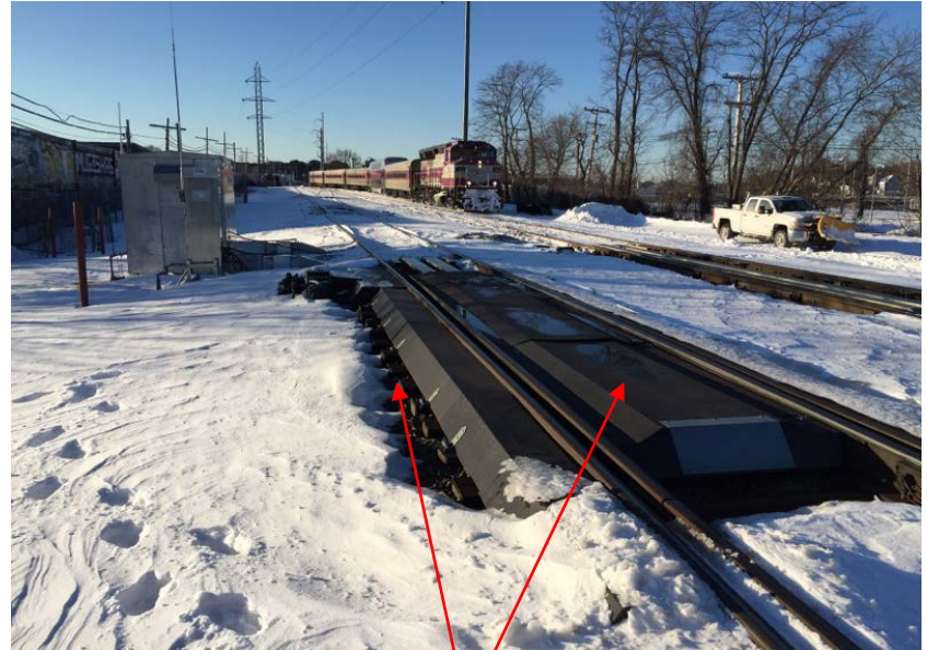
New Gas Heating
