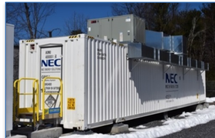
Sterling 2 MW / 3.9MWh ESS Community Resilience Grant
