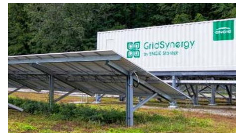
Holyoke 3 MW / 6 MWh ESS Peak Demand Grant
