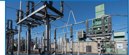
High Voltage Yard
