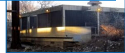
Unit Substation (USS) Equipment
