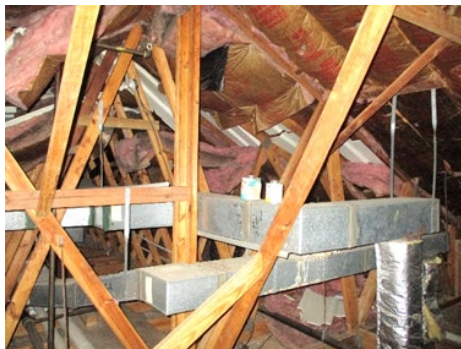
Poor attic insulation
