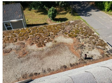
Roof Needing Replacement
