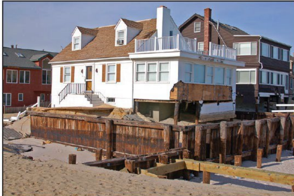
Figure 3-16: Timber bulkhead was overtopped, resulting in lost backfill and damage to the house situated approximately 15 feet landward of the bulkhead (Lavallette, NJ)
